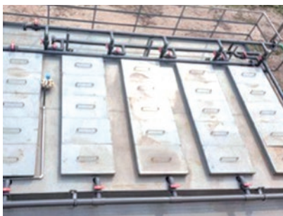
Newly-added advanced processing system
